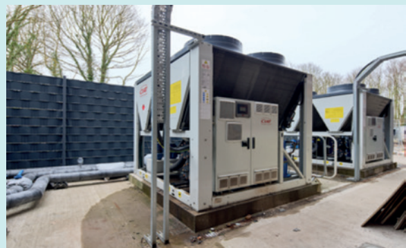
The two external heat pumps
